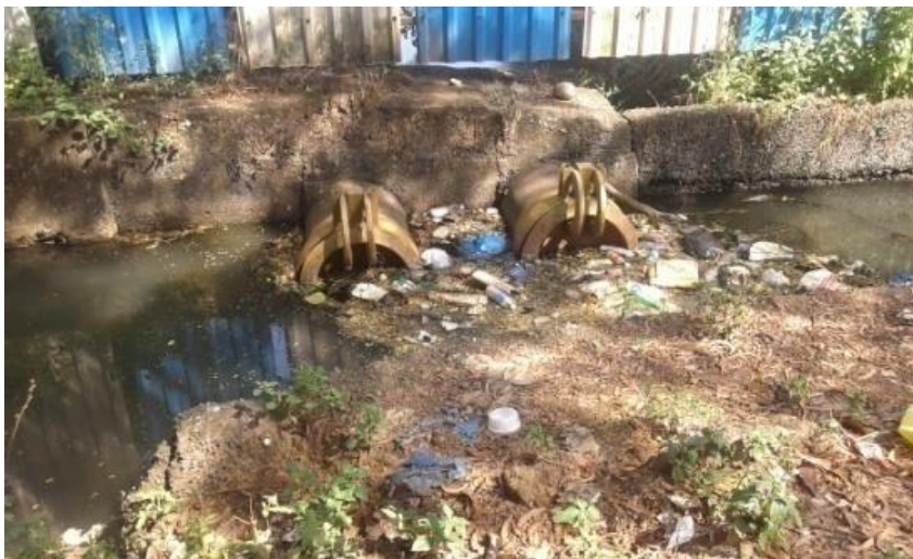
Figure 29: Sluice pipes choked with plastic
