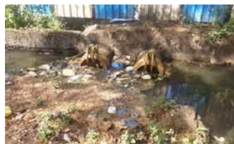
Figure 9: Sluice pipes choked with plastic
